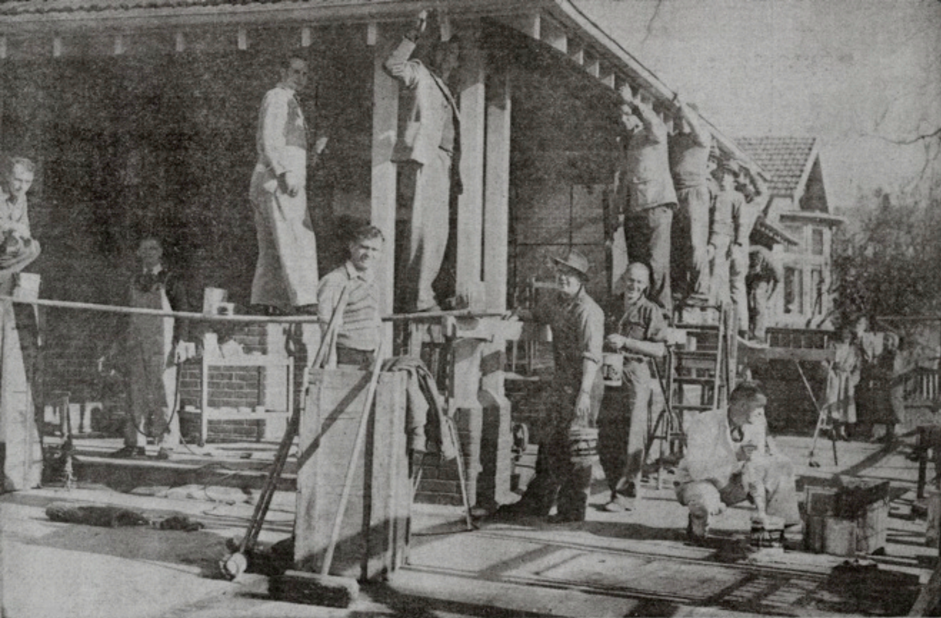
FATHERS' DAY at the Kelsey-Yaralla Kindergarten on Saturday, August 22, 1953, as the men painted the exterior of the building in preparation for the New Zealand Kindergarten Association conference held there later that year.
